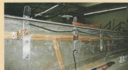
A copper grounding strip for SSB radio is incorporated into the hull moulding
