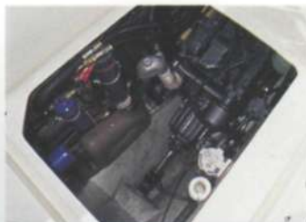
Great engine access, but the unwieldy overhead cover needs hinges and a gas strut
